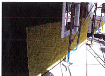
Photo 8: Air Gap. The air gap does not have to be particularly big to be a big deal: 0.375 in. (9 mm). One method of getting the air gap is to use a drainage mat between two layers of building paper. The gap allows redistribution of the moisture in both the stucco and the OSB sheathing. Photo 8 shows the drainage mat installed. Once the mat is installed an additional layer of building paper (not shown) is installed over the mat and then the stucco rendering with lath reinforcing is applied over the top of the additional layer of building paper.
