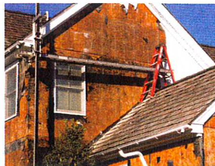
Photo 4: Hardcoat Stucco Failures. Damage is in the field of the wall away from windows.
